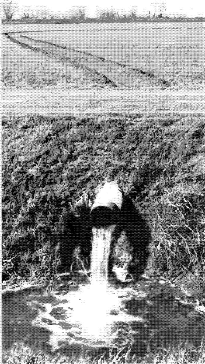
A 12-inch outfall pipe spilling seepage collected from field drain adjacent to the Sacramento River on the Van Ruiten ranch upstream from Kirkville. The flow at the outfall was estimated to be 0.25 cfs.
