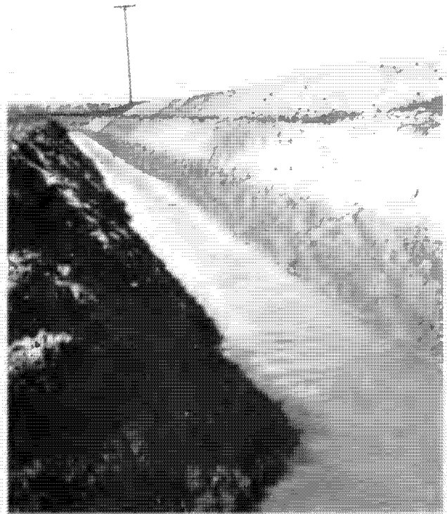
Seepage flowing down the cut-bank of drainage ditch about 1/2 mile away from the Sacramento River on the River Farms property north of Knights Landing.
